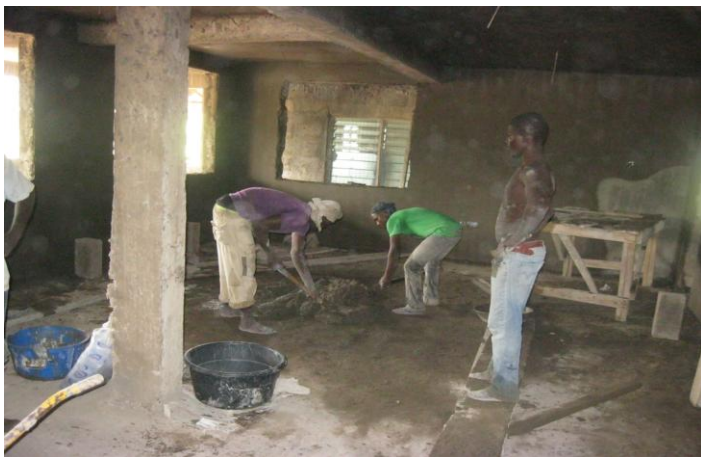
pictured: (left) builders mixing cement to plaster the inside walls of the girls dormitory. (right) the girls bathroom finished tiling work.
