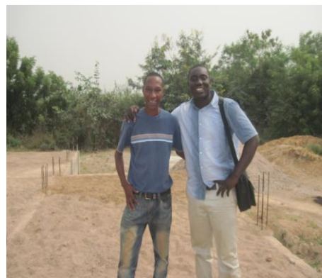
Headmaster Eric Kwame Agoe and building contractor Chief Justice Offin stand on the filled foundation.
