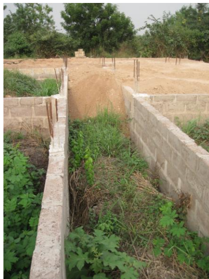
Above: Building foundation is filled with sand. At the end of April only 5 trips are needed
