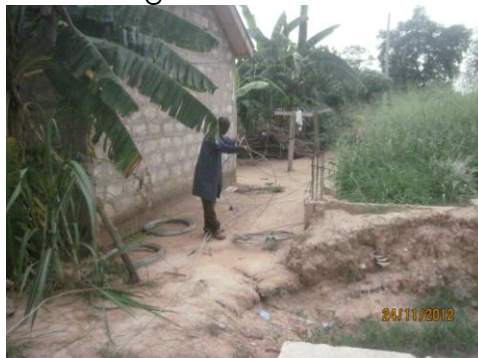
Workers test different areas on MOP land to determine the best place to drill the well
