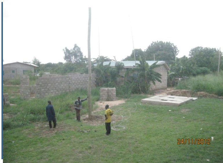
Workers from Ghana Electricity company install light poles and connect wires at MOP building site
