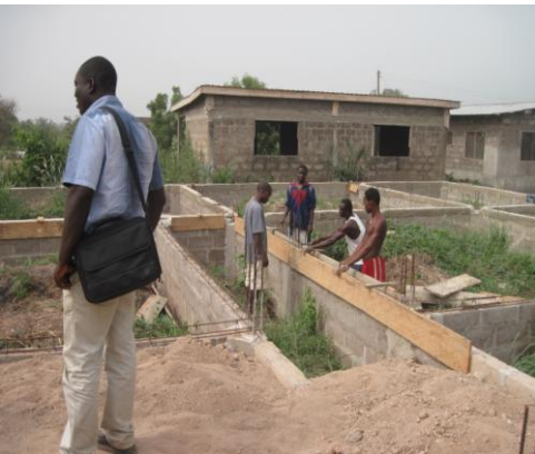
Chief Justice Offin MOP building contractor stands atop one classroom while another gets filled with sand in June 2011.
